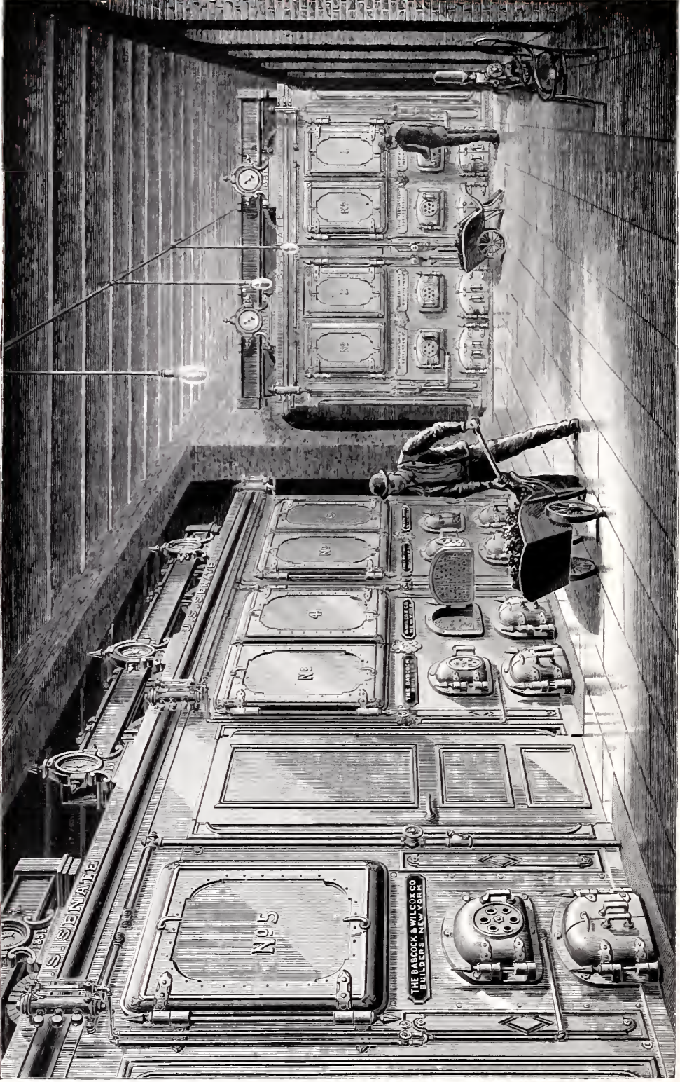
Babcock & Wilcox Boilers in Senato Wing, United States Capitol, Washington, D. C. 312 H. P., erected 1887, 520 H. P., erected 1891.
